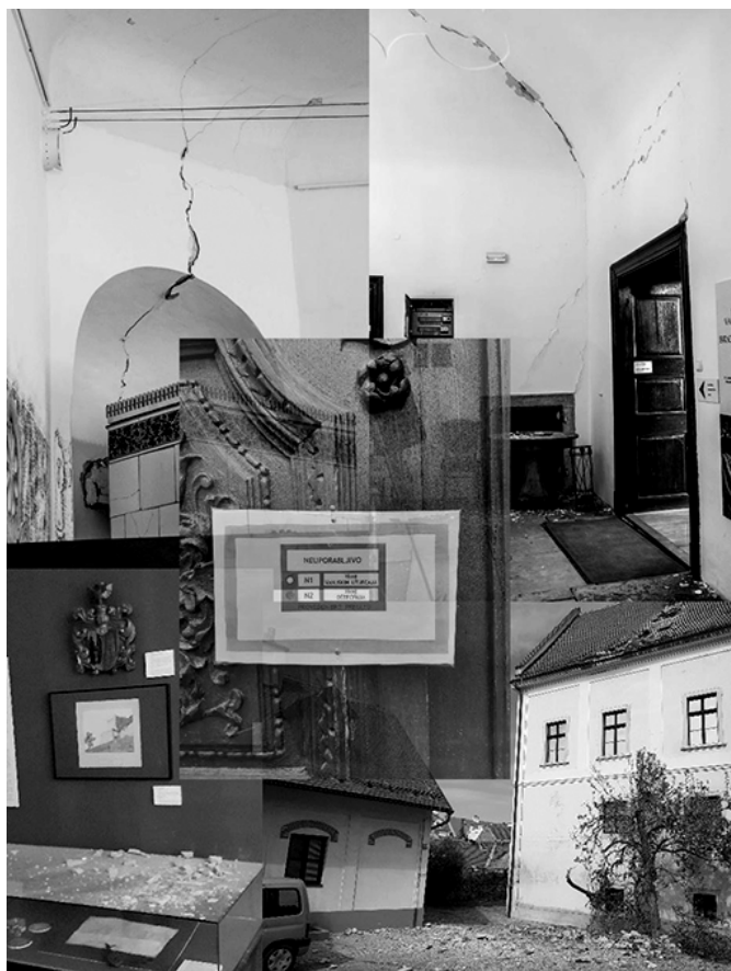
Figure 4. Croatian History Museum - damage caused by the earthquake (Source: Documentation of the Croatian History Museum)
