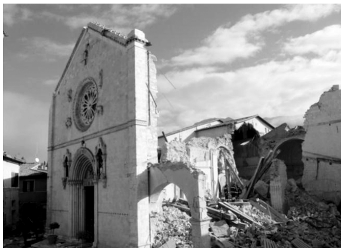
Figure 6. South wall and the facade of the Basilica in Norcia – after the earthquake in 2016. https://uss-sisma2016.beniculturali.it/interventi-sul-territorio/umbria/basilica-san-benedetto-norcia/ (Author: Ministry of Culture in Italy)
